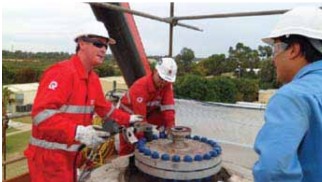
01. Unpacking Mass Transfer equipment for installation 02. Moving Pipework into place under BA for installation 03. Technicians unbolt a Manway with a client supervisor 04. Confined space welding 05. Arc gouging of internal column inserts before removal
